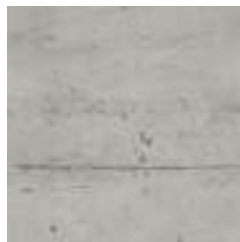
p40 Cold Cracked Concrete
